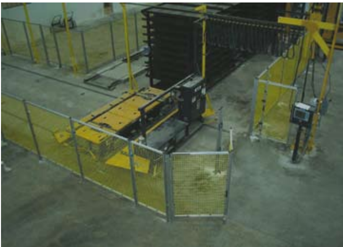
Large bi-fold doors allow forklift access to the kiln area. Note that the operator interface can be located outside of the fenced area for remote control of the rack transfer system.
